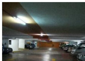
Multi-storey carpark lightings
