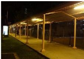
Precinct walkway lighting
